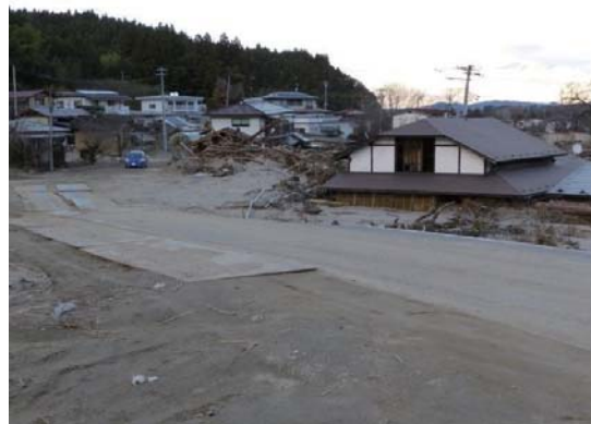
A house half-buried after a flood with a massive amount of sediment hit the area (Marumori Town, Miyagi Prefecture)
